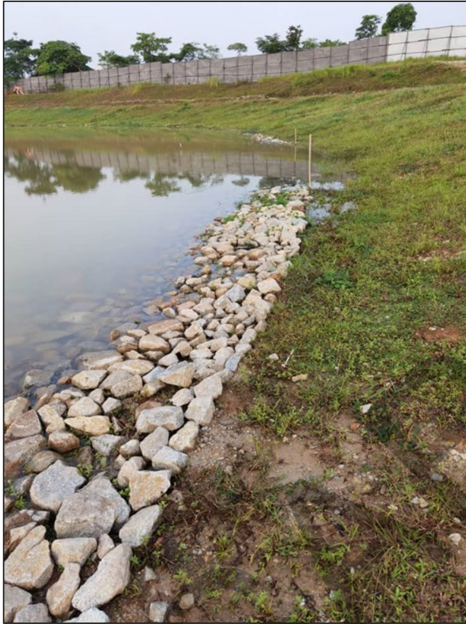
Photo 22 Example of riprap installed at the edge of a lake to trap sediment carried by surface flow.
