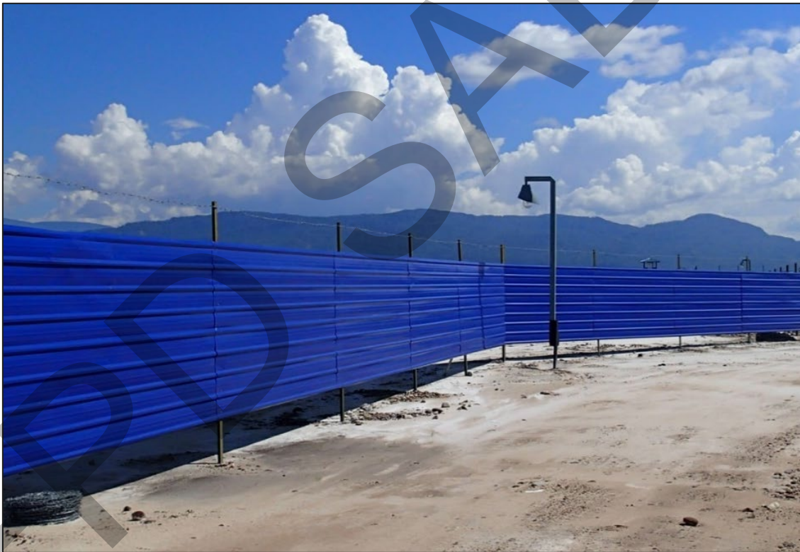
Photo 1 Example of hoarding used to demarcate the active working area within a site.
