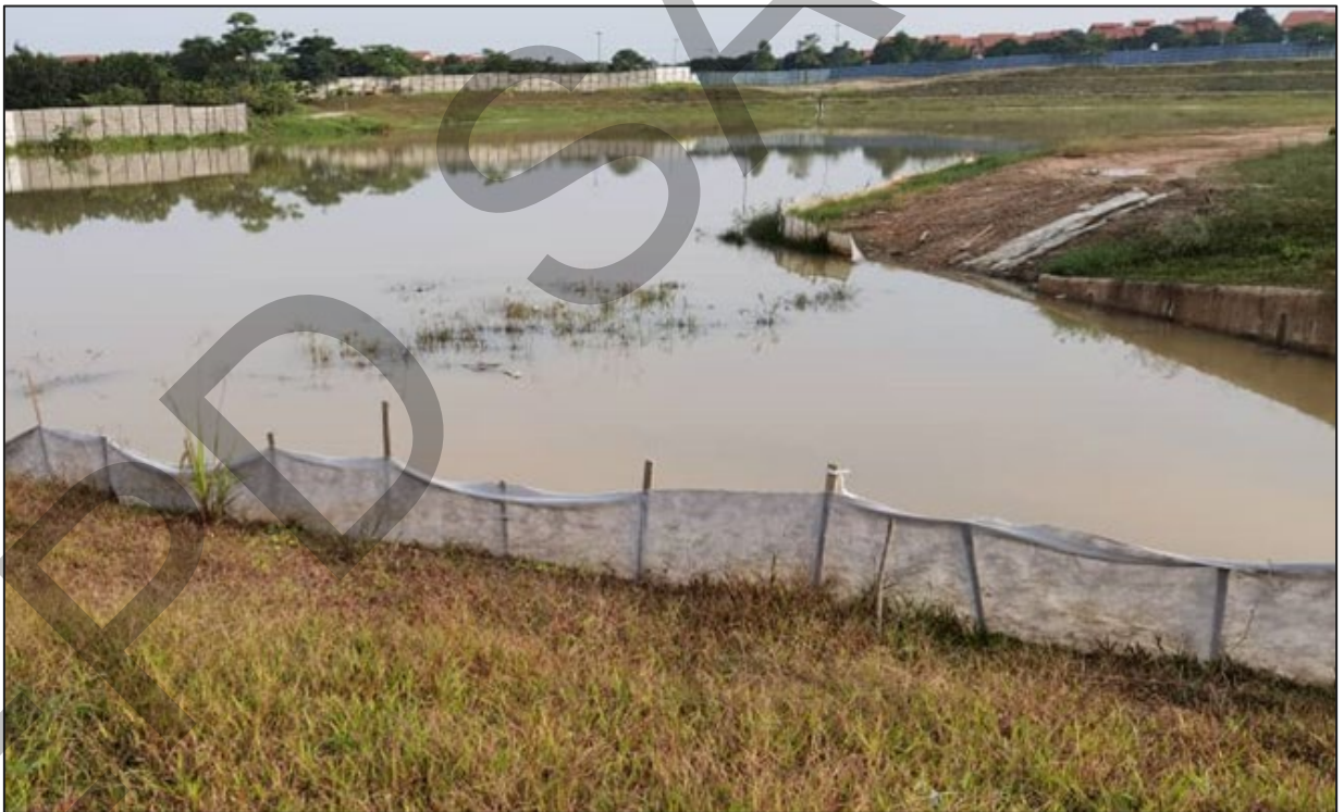
Photo 21 Example of a silt fence installed along the perimeter of a lake.
