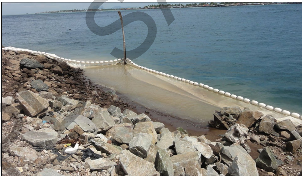
Photo 16 Example of a silt curtain installed at shallow area long the site boundary.
