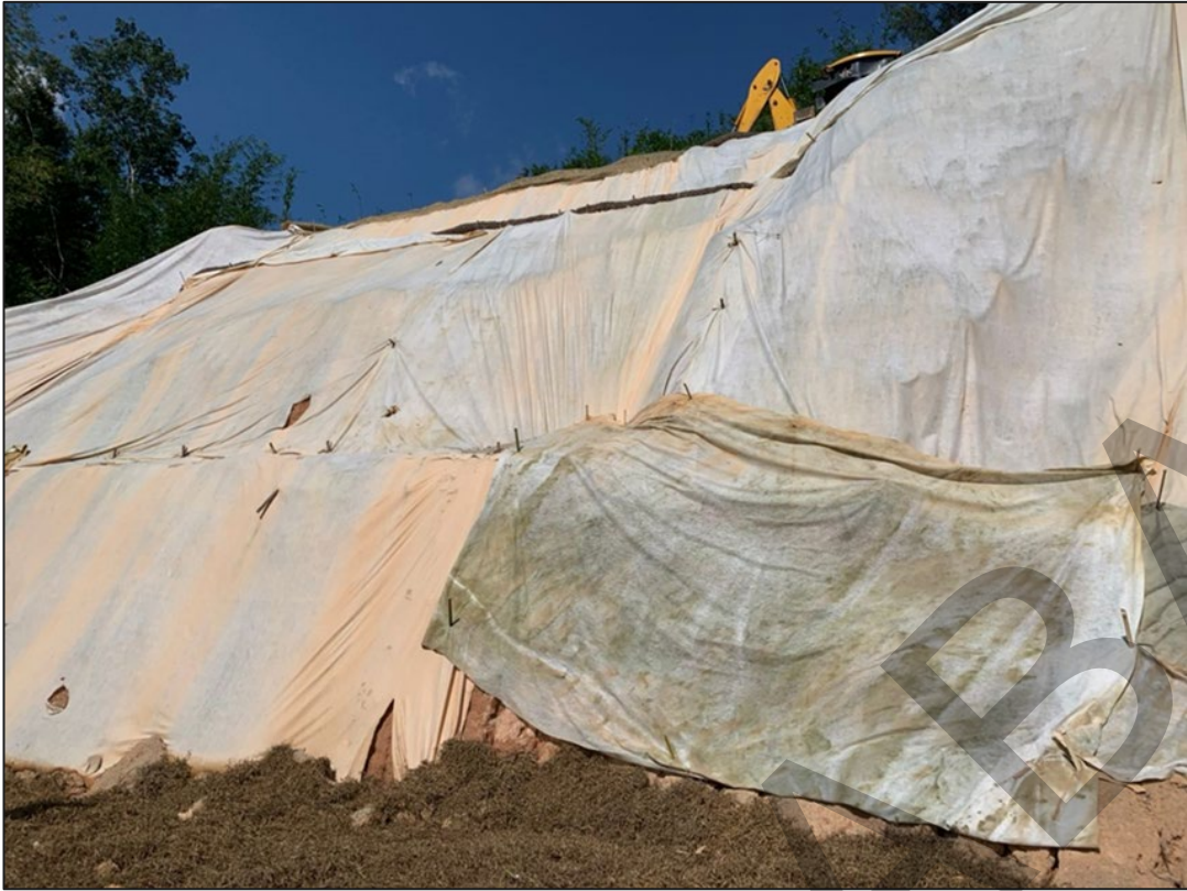
Photo 11 Example of usage of geotextile blanket to cover exposed slope and reduce runoff.
