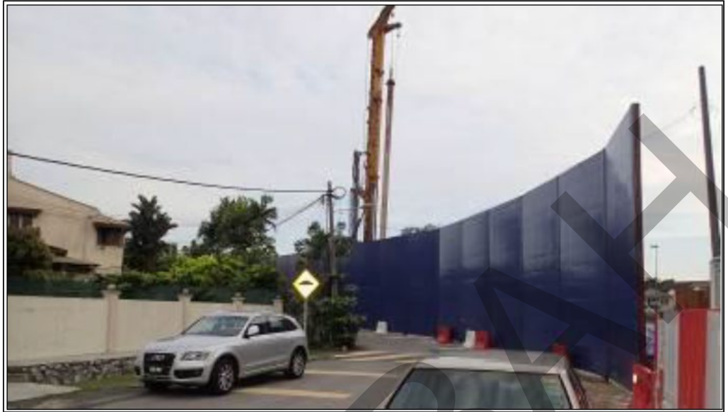
Photo 30 Example of temporary noise barrier using composite panels (Source: Guidelines for Environmental Noise Limits and Control, Third Edition, 2019 (p. 103), DOE)
