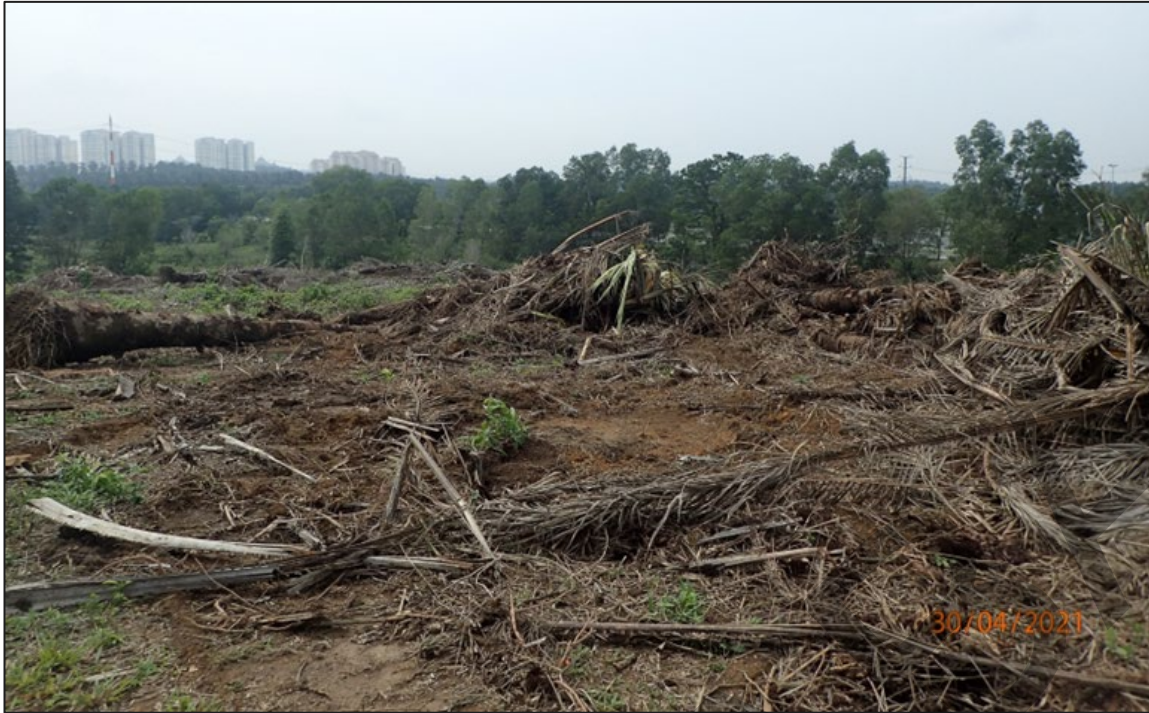
Photo 6 Biomass or mulch can be applied on exposed soil ground to reduce erosion runoff at site.
