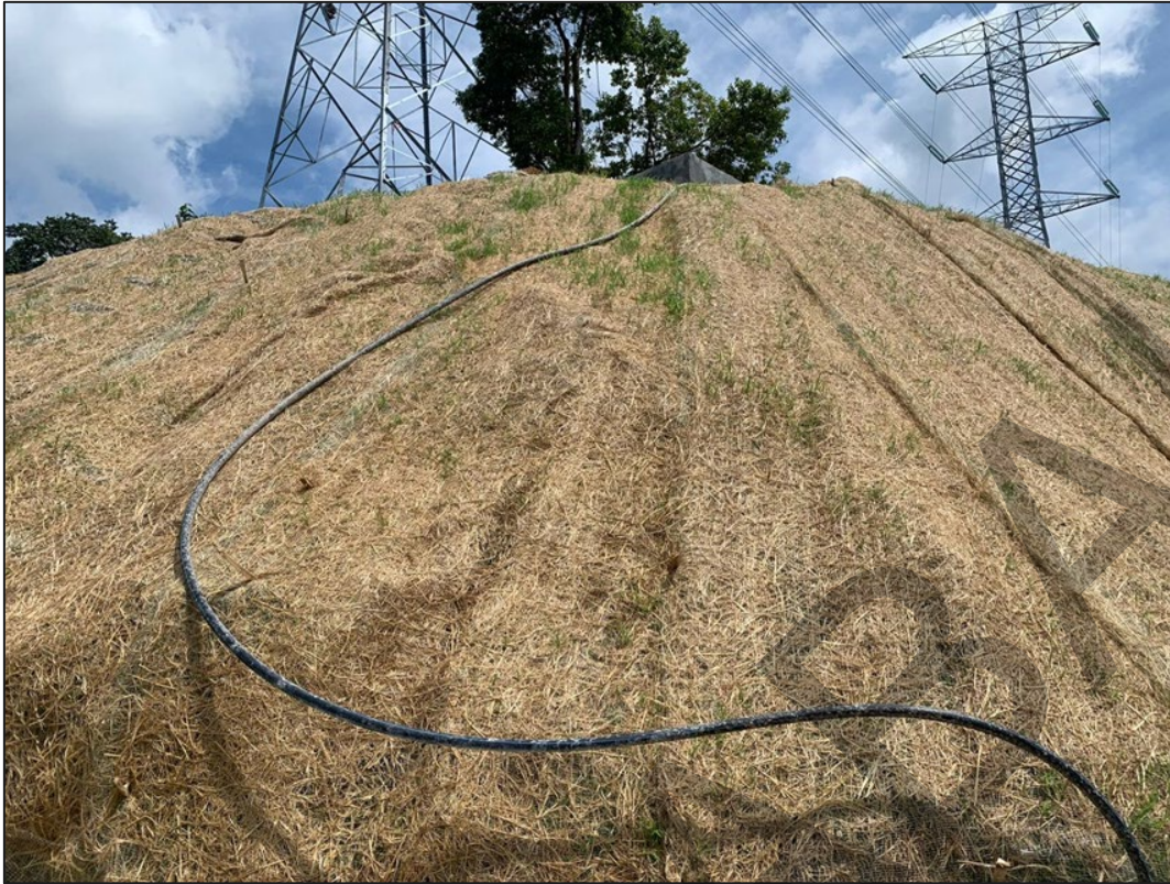
Photo 13 Example of roll erosion control blanket (Organic mulch materials) anchored on the slope surface to control erosion and stabilise slope.
