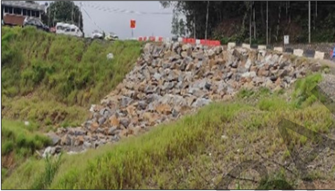
Photo 24 Example of riprap slope protection after a landslide event.
