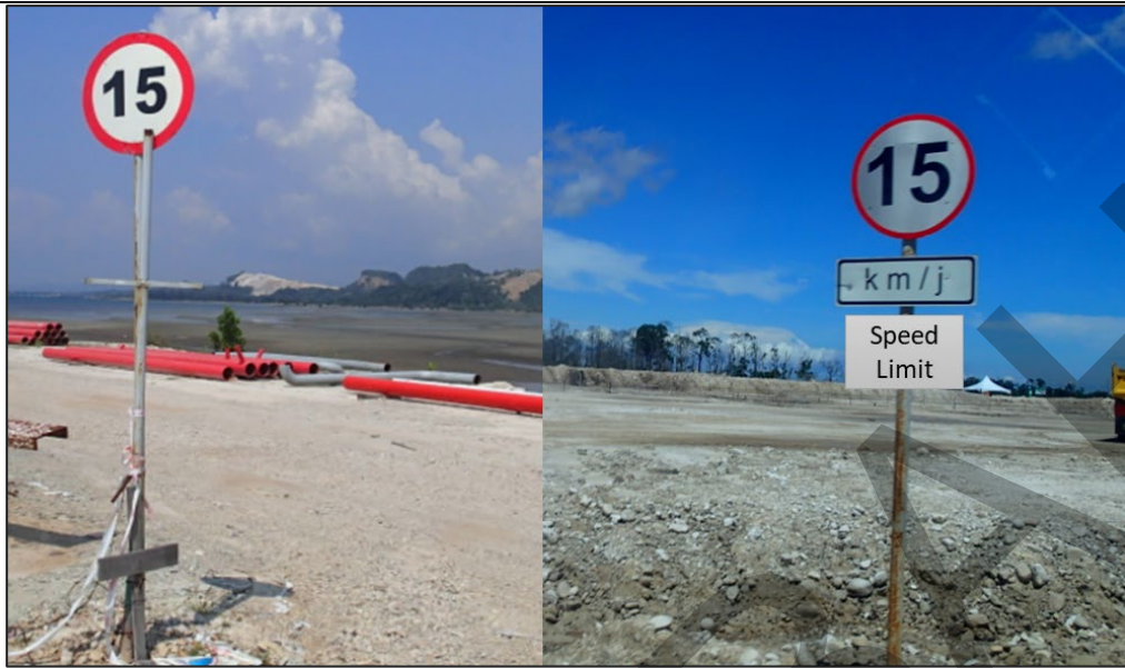
Photo 37 Example of speed limit sign installed at construction site.
