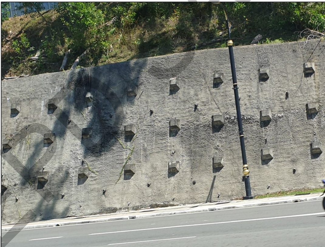
Photo 25 Example of soil retention structure / reinforced concrete retaining walls using the soil nail method.
