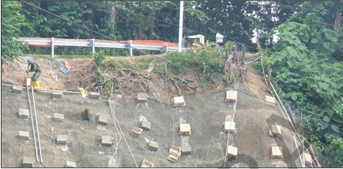
Photo 28 Example of on-going construction of rock slope stabilisation protection (i.e., soil nail and netting method) to stabilise slope after landslide event.
