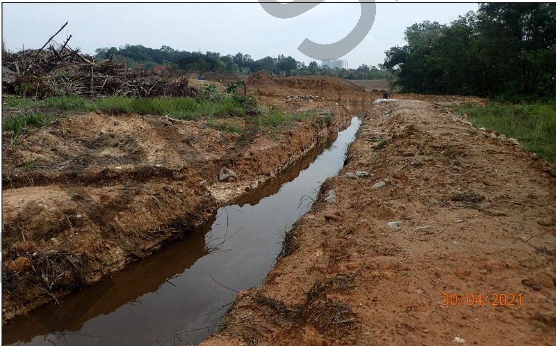
Photo 7 Example of temporary perimeter earth drain constructed to divert runoff or channel water to silt trap / sediment basin / sediment pond / sump.
