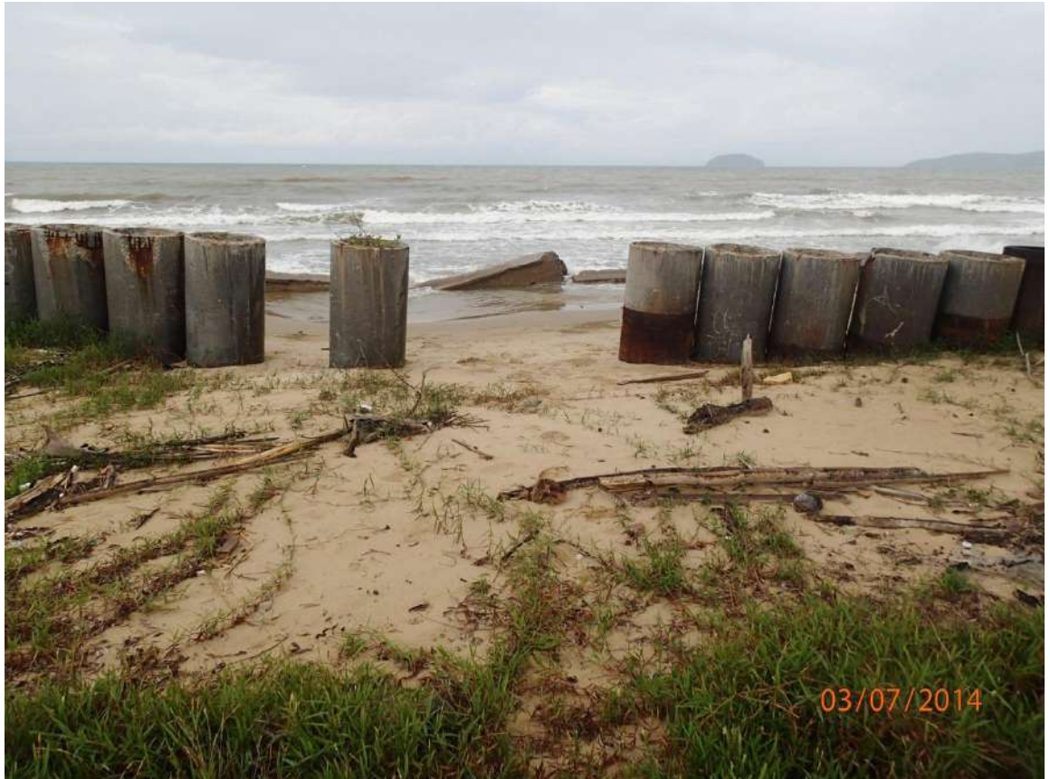
Photo 3.5 Erosion extending behind the primary line of defence and through the second line of defence (concrete piles)
