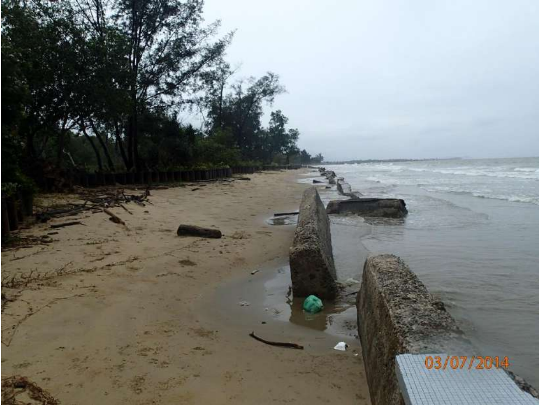
Photo 3.11 Submerged concrete structures a hazard to swimmers and other beach users
