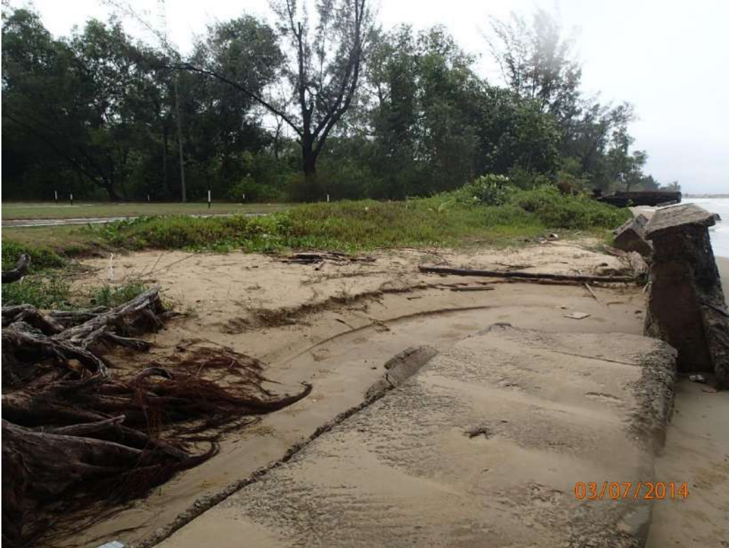
Photo 3.4 Erosion extending behind the line of the existing concrete sea wall
