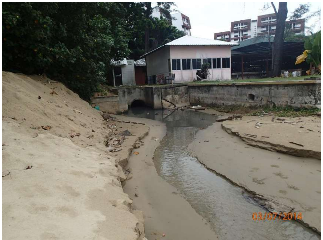
Photo 3.8 Drain outfall discharging onto the beach north of the Sugarbun
