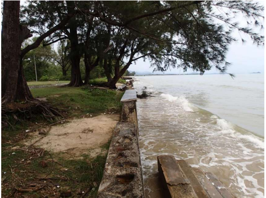
Photo 3.2 Sea encroaching right up to the old seawall at high tide and covering the amenity beach
