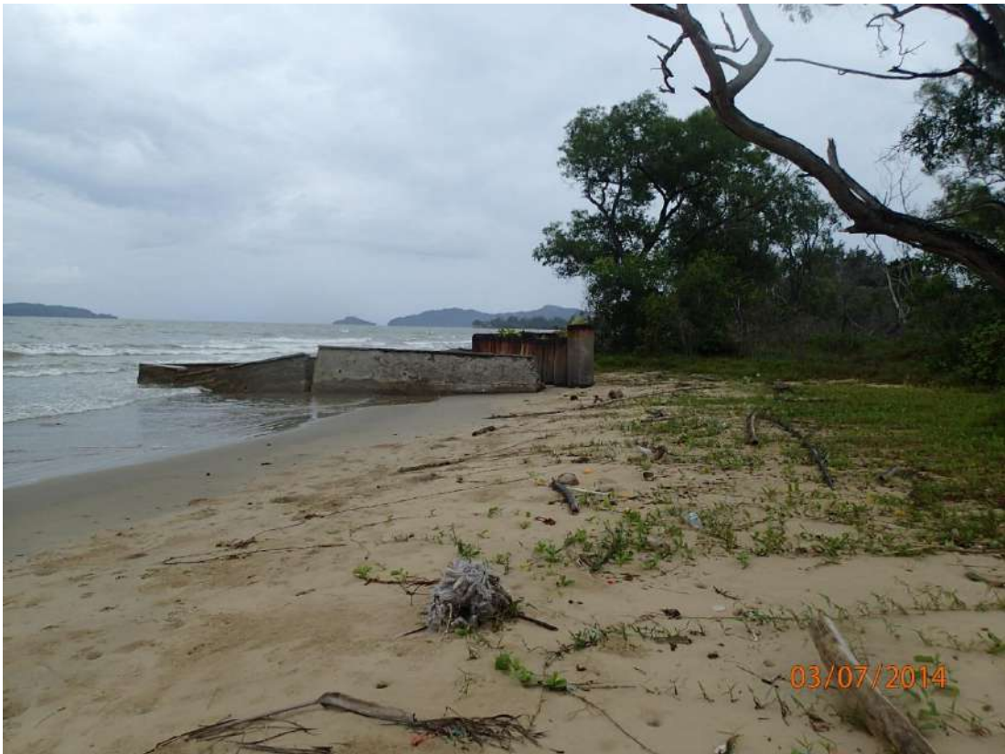
Photo 3.12 At high tide and with rough seas access along the beach is cut off
